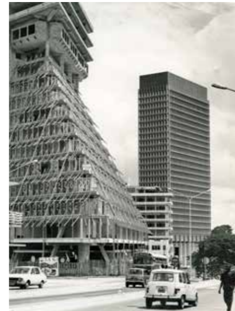
"The Pyramid" under construction. Designed by Italian architect Rinaldo Olivieri and built from 1968 to 1973, this imposing edifice in the Plateau business district came to symbolize the 1980s economic boom in Côte d'Ivoire. Abidjan, 1972.
